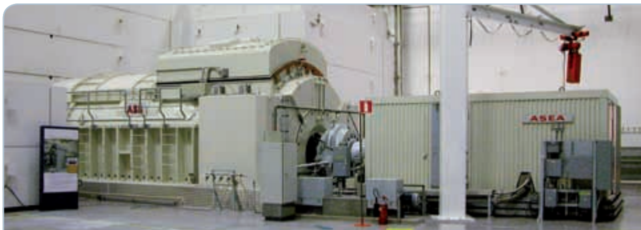
Generator and exciter.
