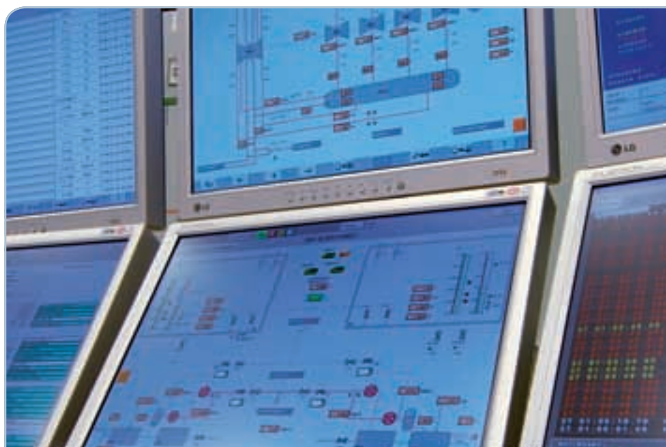
Turbine control displays. Using the simulator, operators can practise controlling the power plant without interfering with its actual normal operations.
