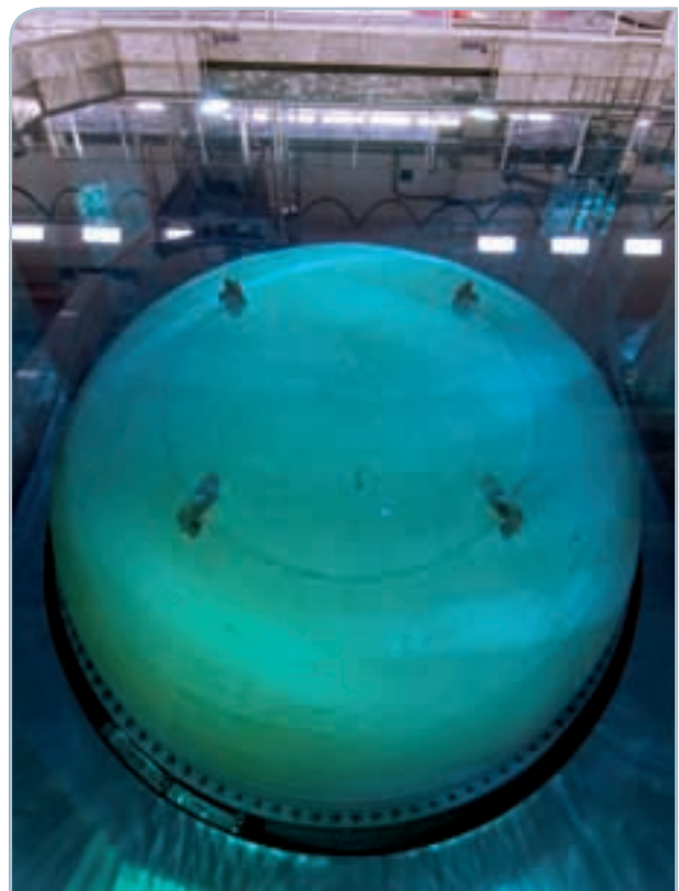
The reactor steel cover is fixed with 120 bolts. The cover is sealed with O-ring seals.
