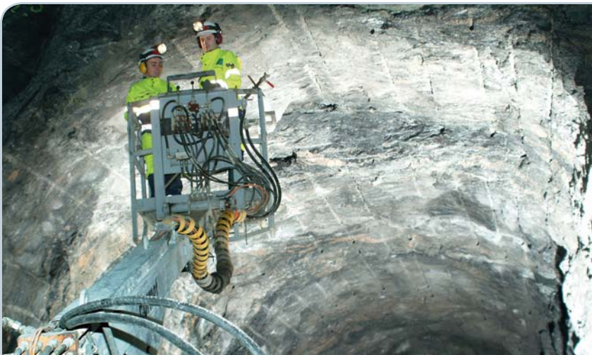
The excavation work for the tunnel into Onkalo, the research facility for the spent fuel repository has reached the depth of 400 metres. The tunnel is about 4 kilometres long.
